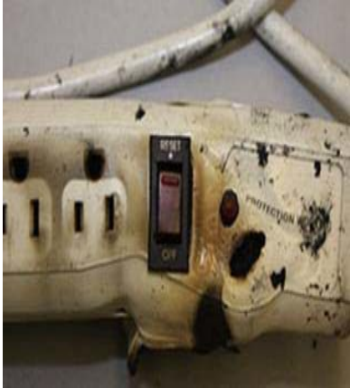
Overloaded power bar
