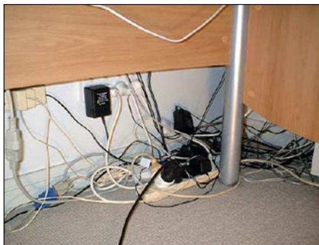
Serious electrical hazard
